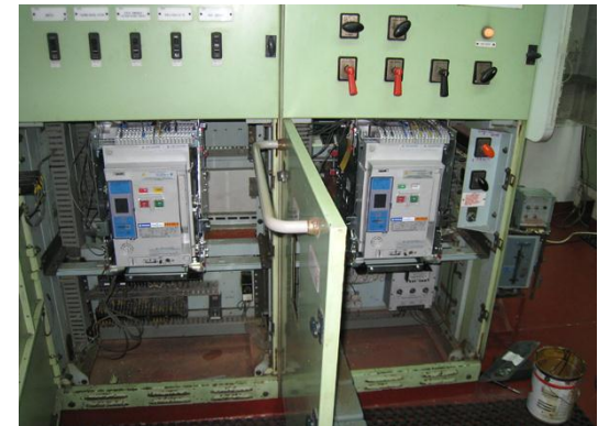
New TemPower2 installed
