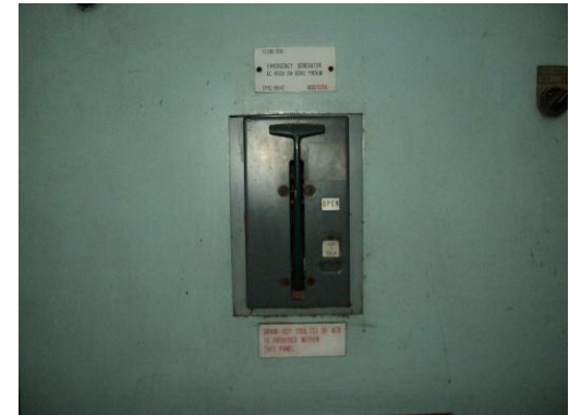
Old type breaker AH16B in the panel
