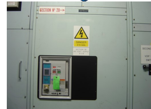
After: Retrofit ACB, protection relay with LCD
